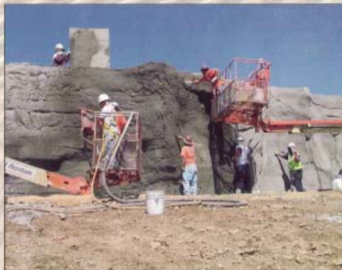
Shotcrete sculpted rock wall is installed and finished by sculptors and chromatic artisans.
